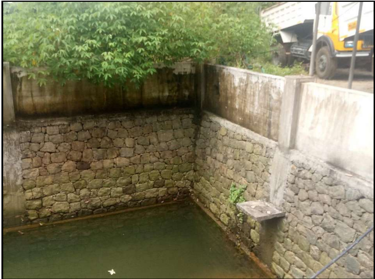
Photograph showing the rain water harvesting tank
